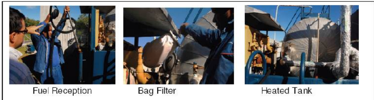
Picture 5.4: Biofuel Installation Ouvea, New Caledonia
