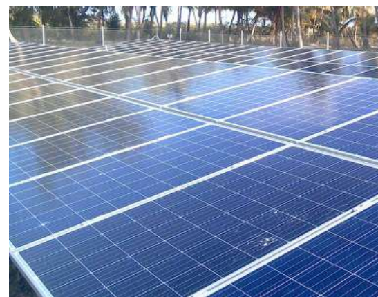
Solar panels for power in the outer islands. (source: www.mise.gov.ki)
